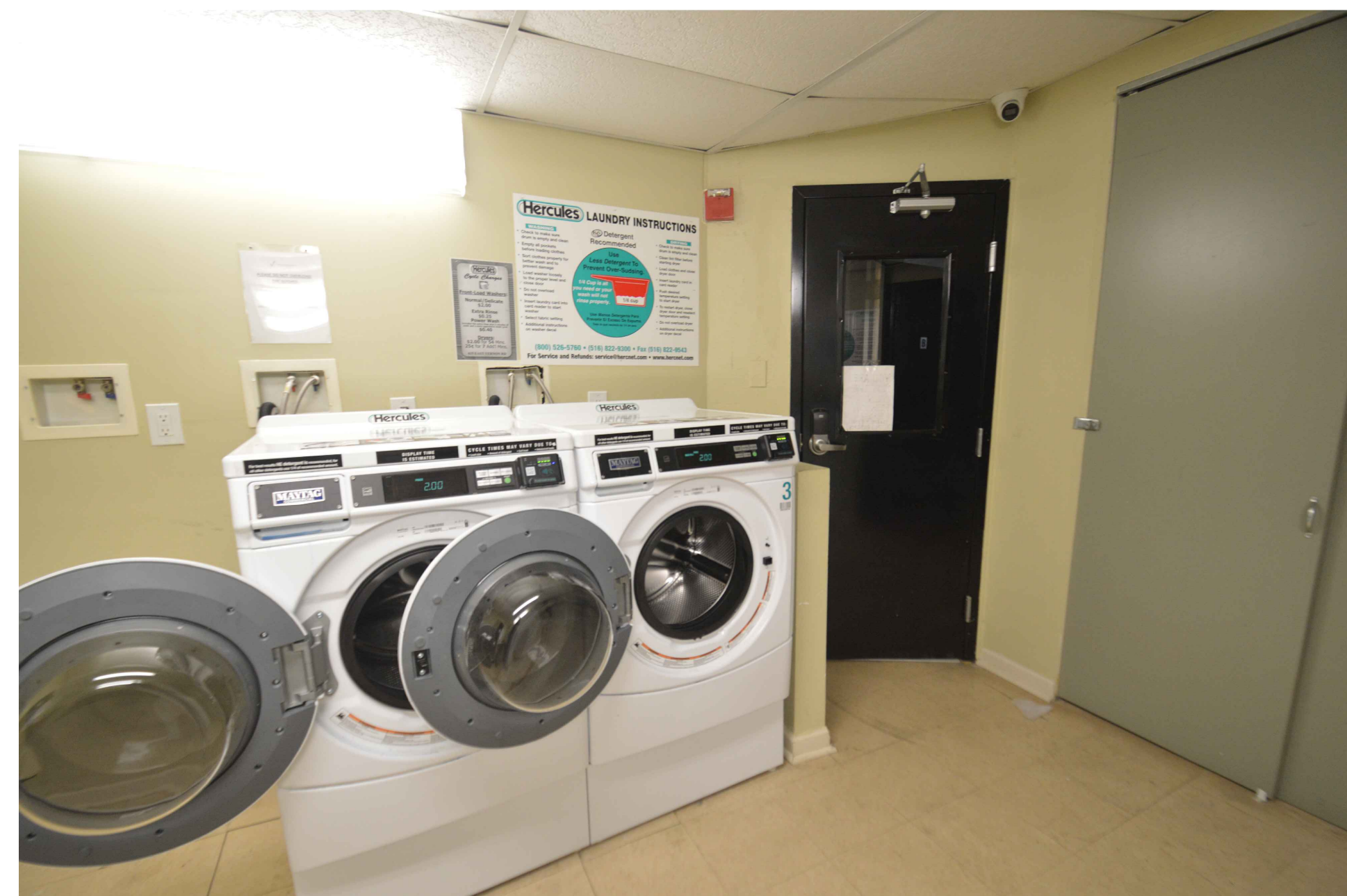
Shared Laundry Room
